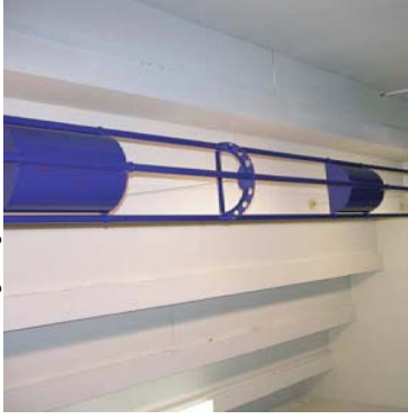
Concourse lighting fixture:
