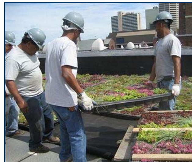
Installation of a Green Roof at the Betty Ruth and Milton B. Hollander Foundation Center
