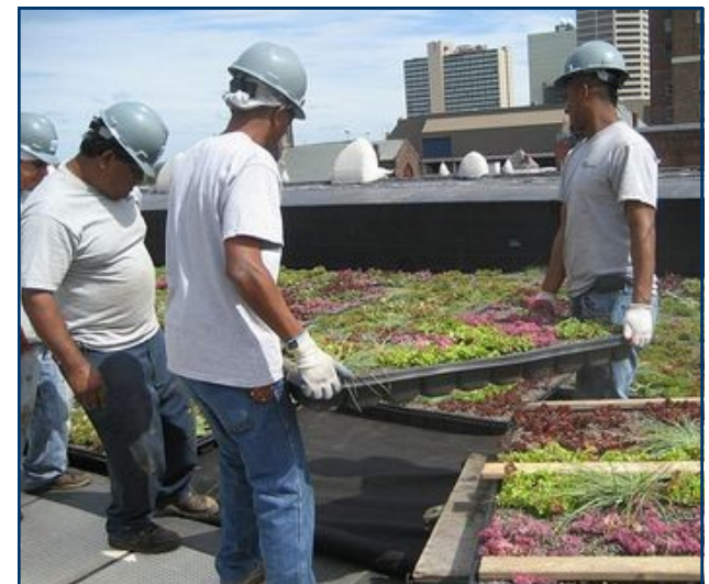
Installation of a Green Roof at the Betty Ruth and Milton B. Hollander Foundation Center
