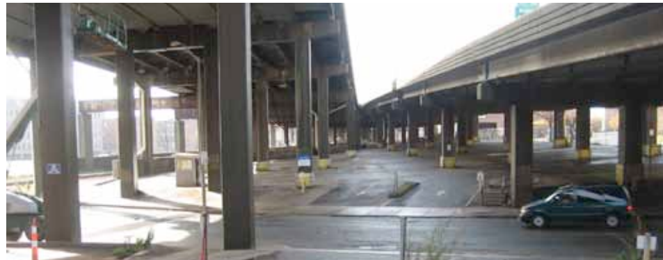
The Viaduct structure is nearing the end of its useful life and will need to be replaced.
