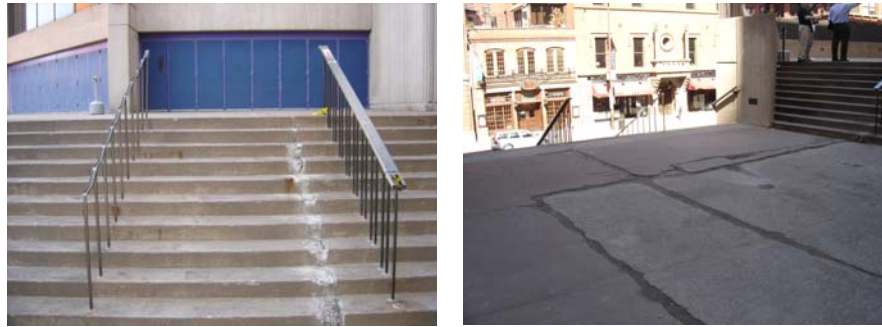
Southwest corner of the building used as a smoking section. There is significant wear and delamination of the concrete steps and pads
