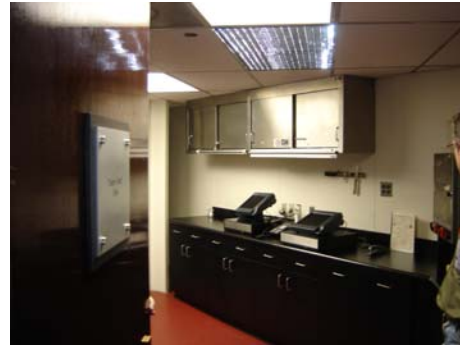
Pantry on the suite level used to service the suites is in good condition
