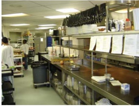
Kitchen on suite level has enough space to accommodate large scale cooking for premium areas and catering activities
