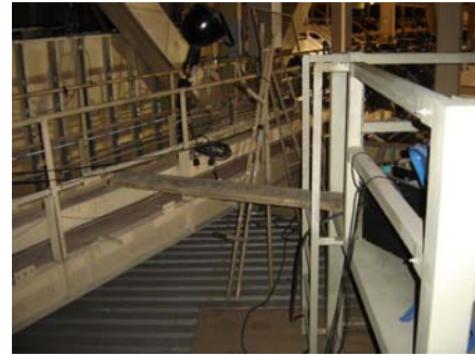
Spotlight platform at SW corner – 2x8 inch board used to access platform from the catwalk
