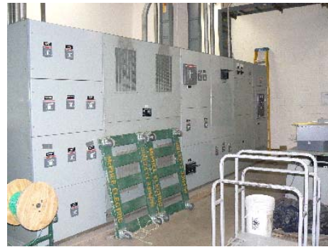
Note the storage of event equipment and the dust / grease residue coming out of the vents in this pane
