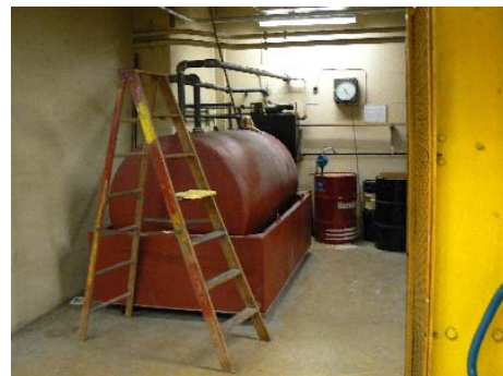
Fuel Storage Tank
