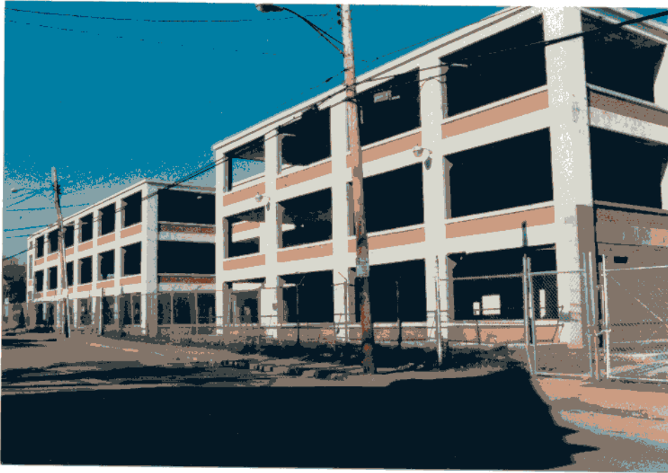
Veeder Place at the northern border of Asylum Hill is currently undergoing rehabilitation.
