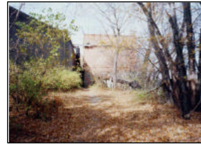
Pumping Station on the Connecticut River
